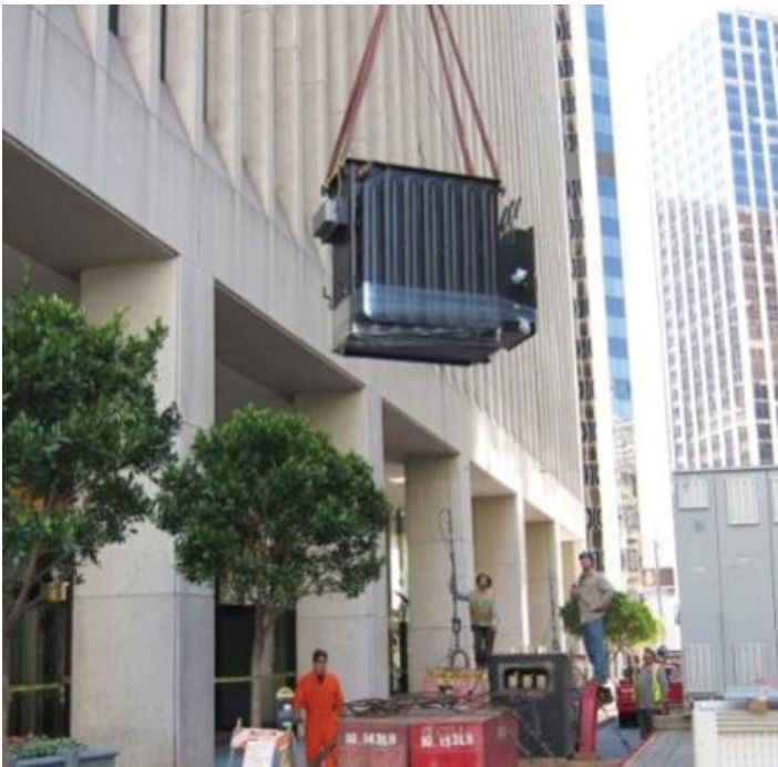
High-Rise Dry-Type Installation
