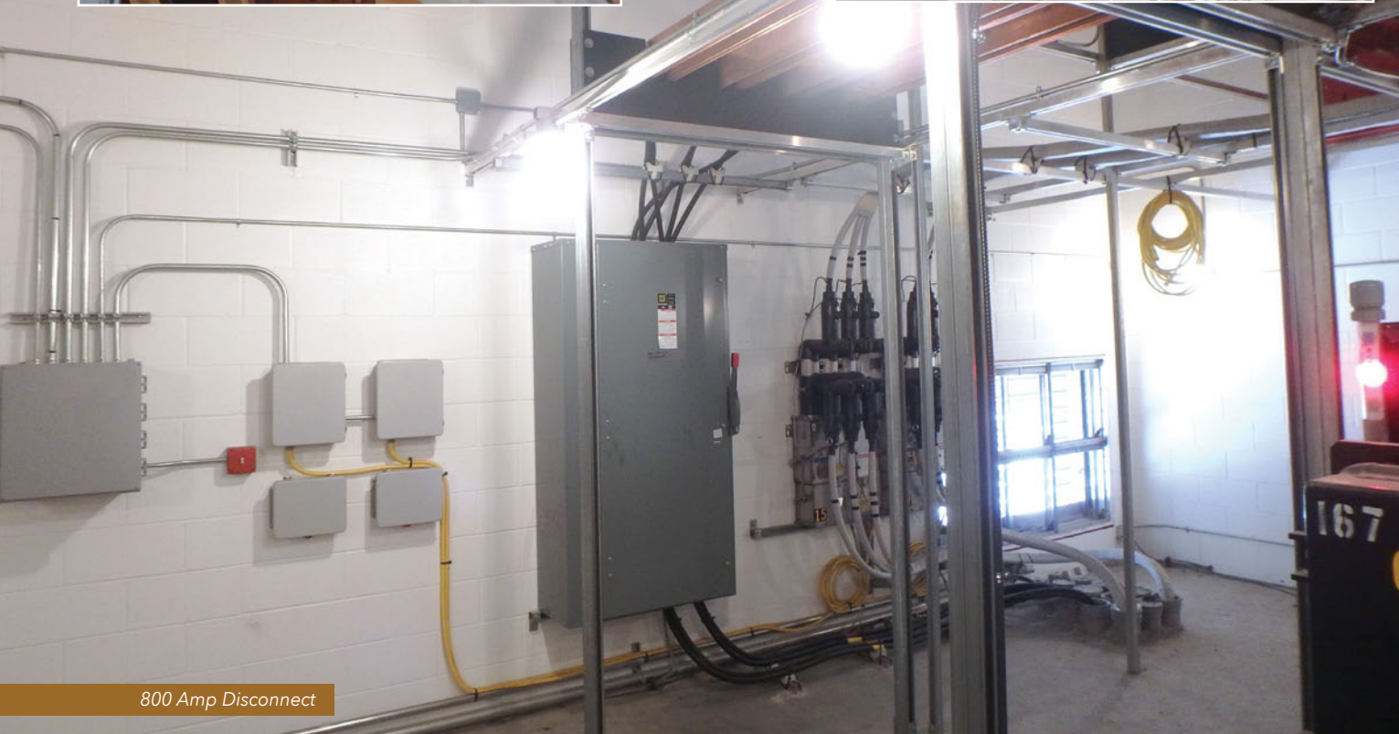
800A Disconnect connected to energized bus
