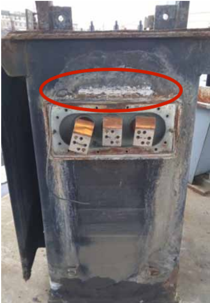
Consumed throat anode with tank material intact
