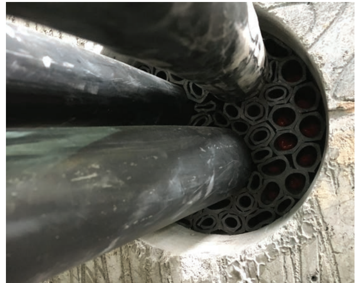
Cables supported and separated
